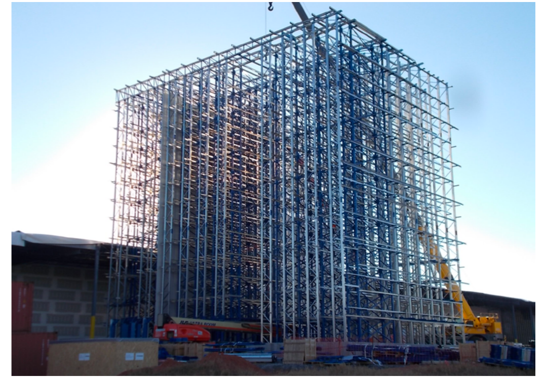
AUTOMATICO AUTOPORTANTE AUTOMATED CLAD-RACK WAREHOUSE
